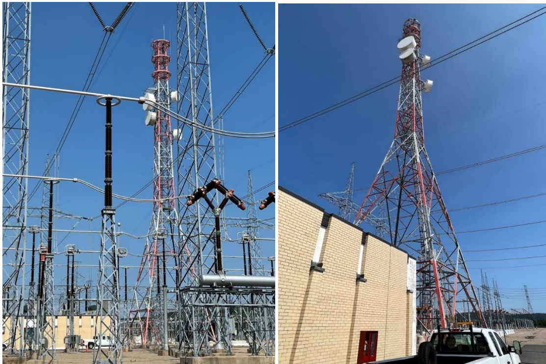
Figure 1 : Telecommunication tower in a 735 kV substation, the antenna are placed above 38m. Source Hydro-Québec
