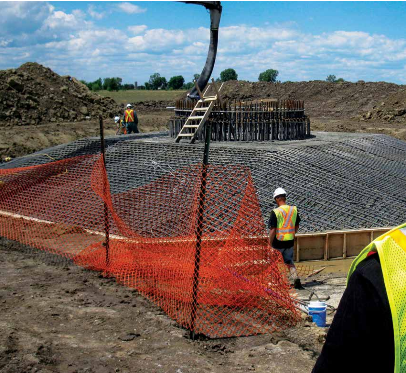
Brookfield employees wearing the proper safety gear as they complete work on the jobsite. Photo courtesy of Brookfield Renewable Energy Group.
