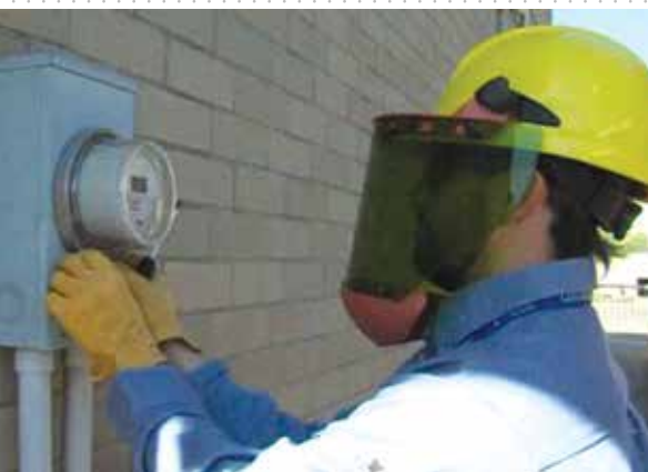
Employee installs an automated meter in Medicine Hat, Alberta. Photo courtesy of the City of Medicine Hat.
