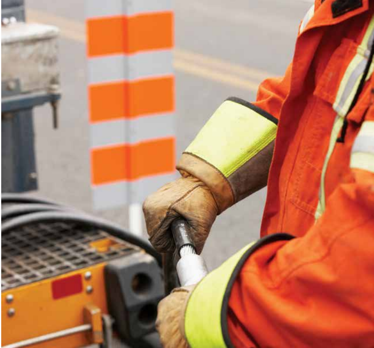
Hydro-Québec distribution lineman demonstrates transferring a pole with an isolating switch. The work is performed with voltage according to the Live Working Standard contact method (with insulating gloves). Photo courtesy of Hydro-Québec.
