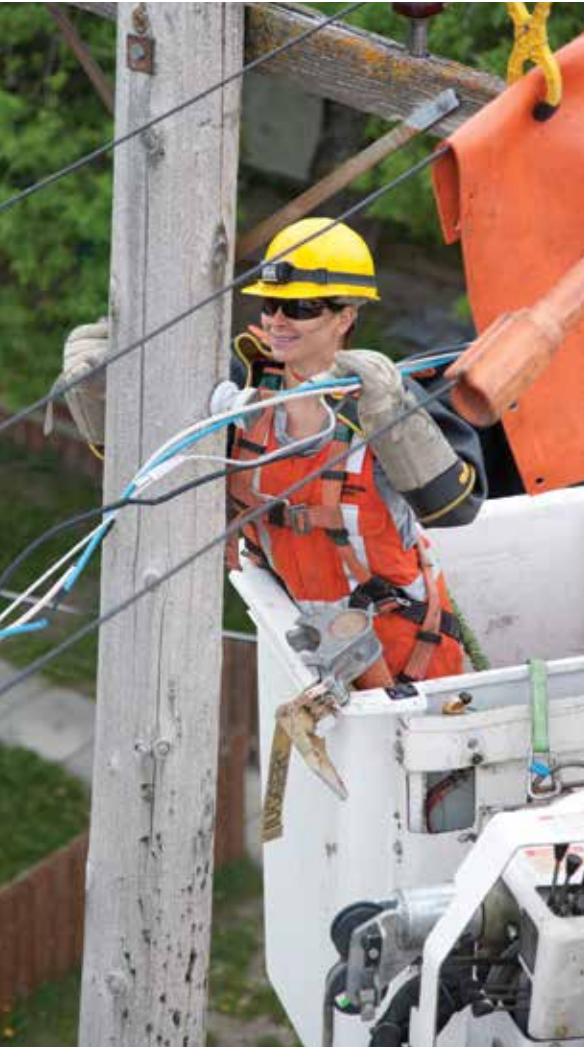
Power line worker Jessica Hadfield safely repairing a line. Photo courtesy of Manitoba Hydro.
