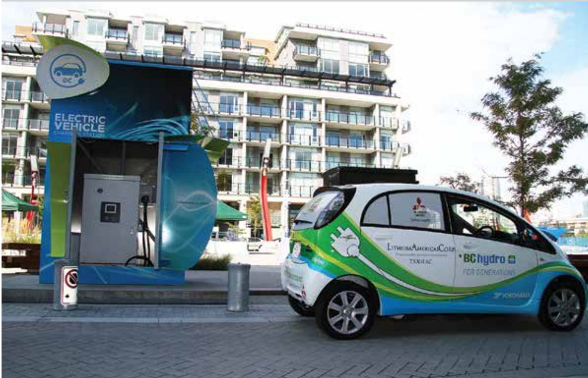
Electric vehicle Direct Current fast charging demonstration by BC Hydro. Photo courtesy of BC Hydro and Power Authority.
