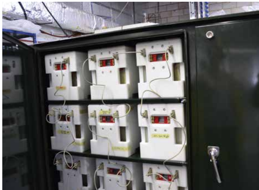
Toronto Hydro's community energy storage system was developed with a lithium-ion battery solution used for distribution grid applications. It consists of batteries, controls, and communication systems that interface with the grid and was made possible through funding in innovation. Photo courtesy of Toronto Hydro Corporation.
