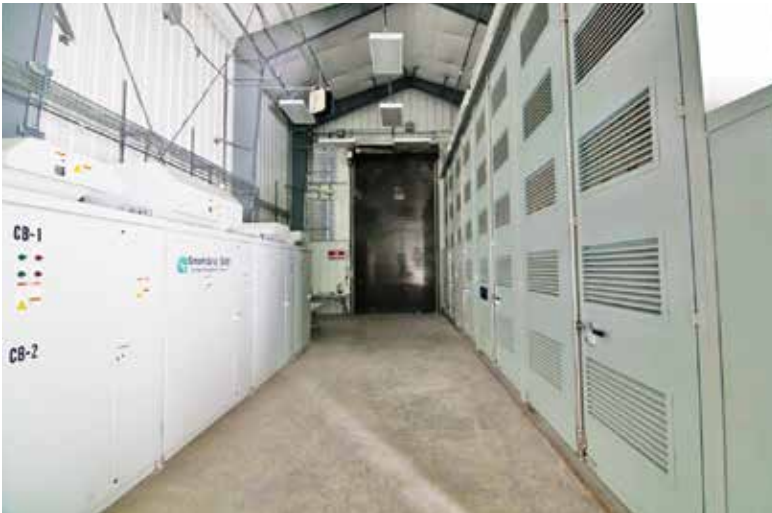
A view of the interior of BC Hydro and Power Authority's Field energy storage facility. Photo courtesy of BC Hydro and Power Authority.
