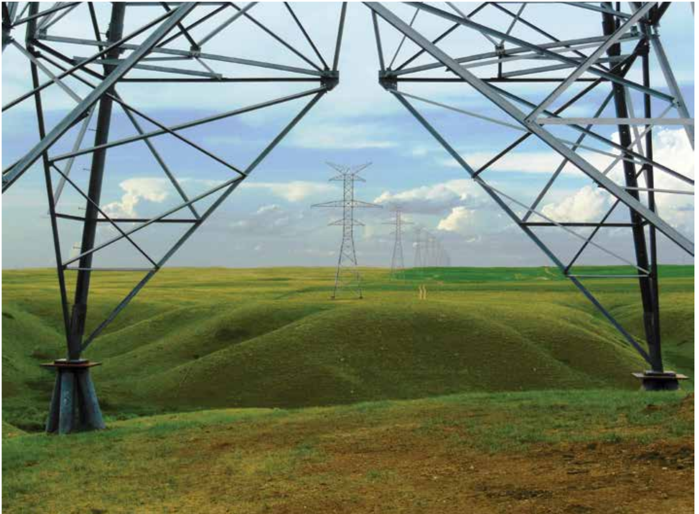
AltaLink's Bowmanton to Whitley Transmission Project—a 240 kV transmission line from east of Medicine Hat to South of Whitley—was built on screw pile foundations. Photo courtesy of AltaLink.
