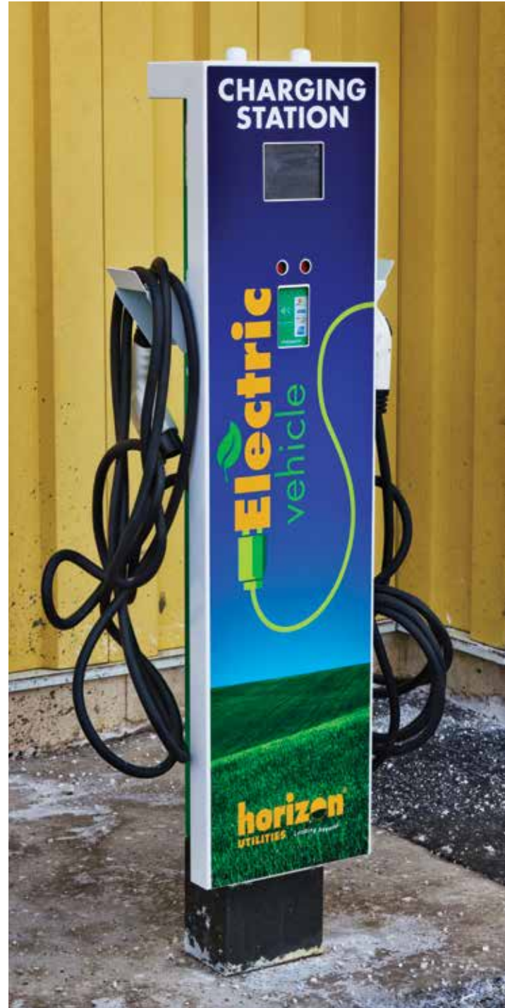
Horizon Utilities’ electric vehicle charging station. Photo courtesy of Horizon Utilities Corporation.
