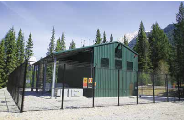
A view of the exterior of BC Hydro and Power Authority's Field energy storage facility. Photo courtesy of BC Hydro and Power Authority.
