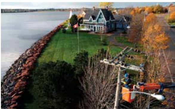
Power line technician ensure power reliability. Photo courtesy of Maritime Electric Company Limited.
