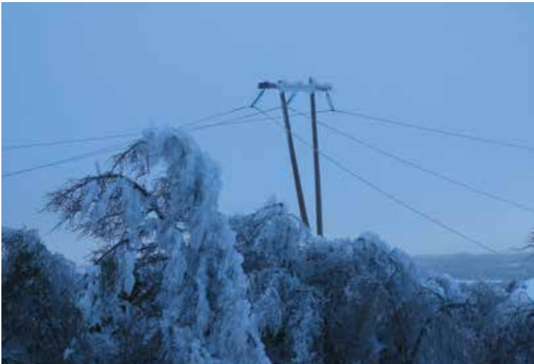
Storm related damage caused by freezing rain in Newfoundland. Photo courtesy of Newfoundland Power Inc.
