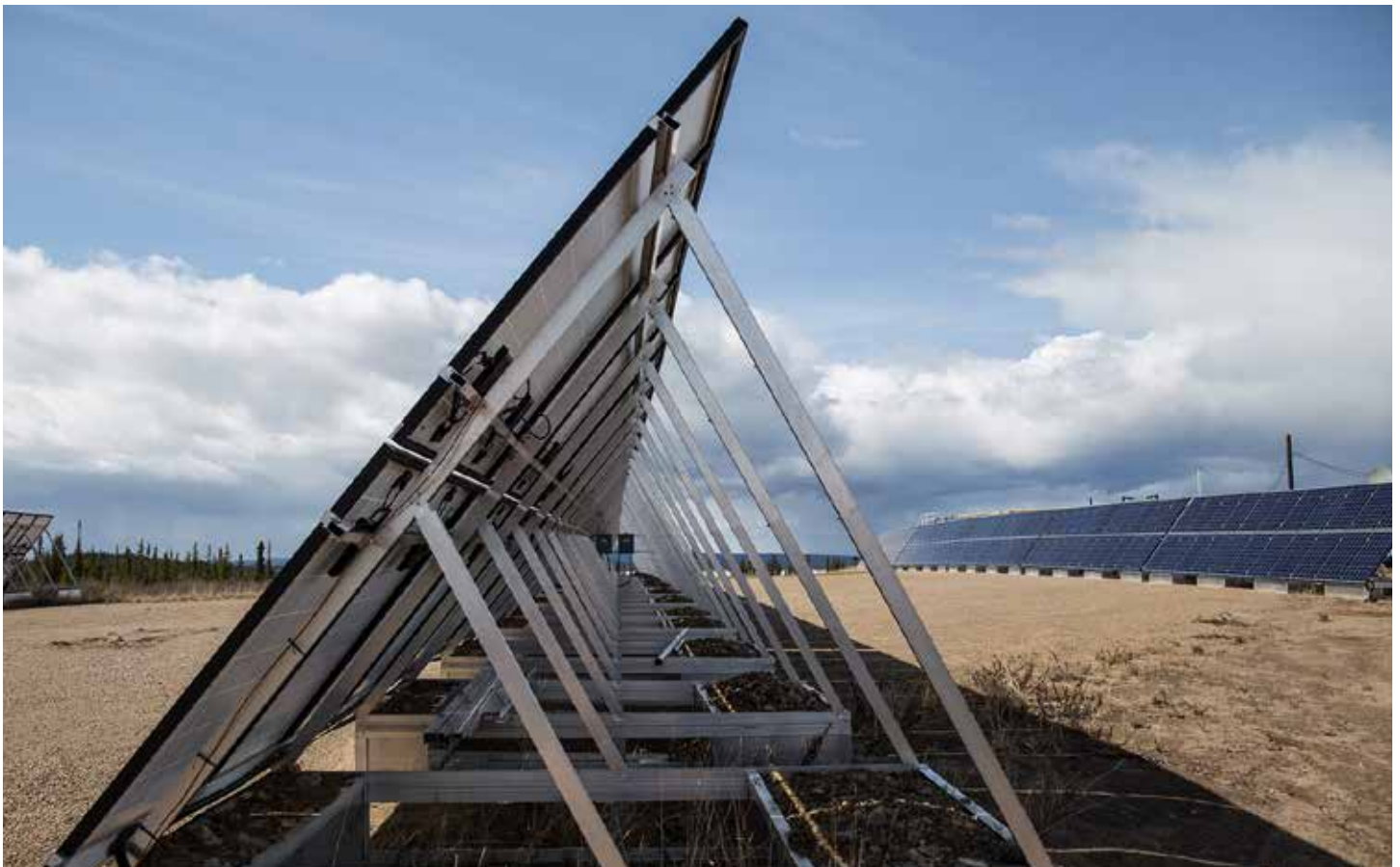
Photo courtesy of Northwest Territories Power Corporation.
